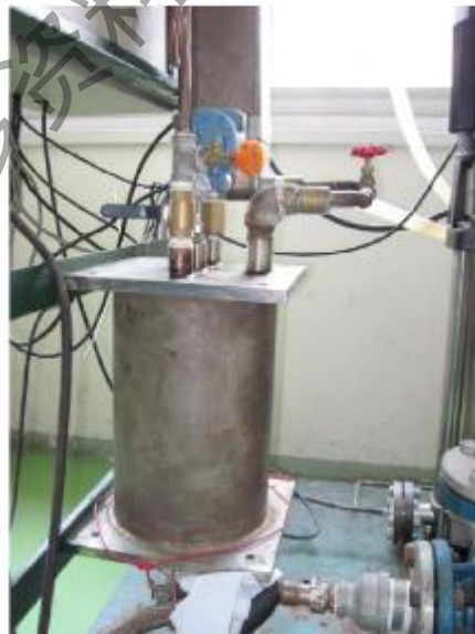
图 5-8 储液罐 Figure 5-8 Tank
