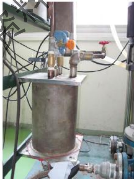
图 5-8 储液罐 Figure 5-8 Tank
