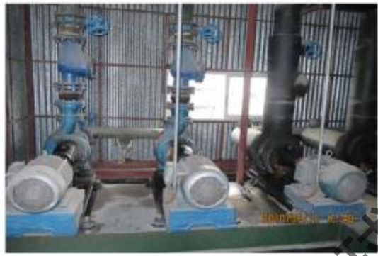
图 6-15 冷却水泵、冷冻水泵 Fig. 6-15 Condensed water and cooled water pumps
