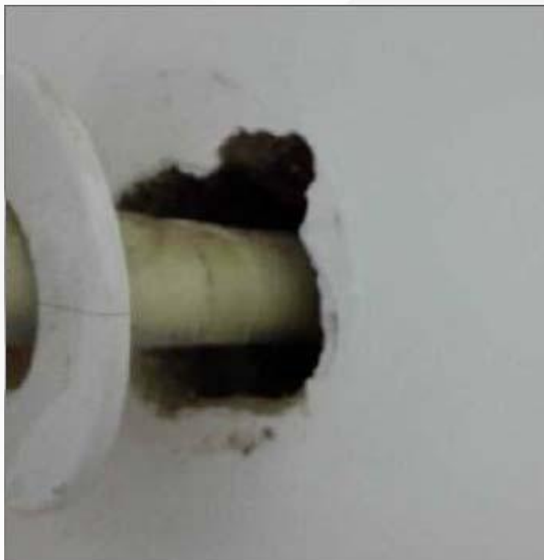
墙孔内未加塞胶泥
