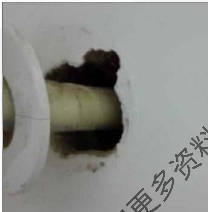
墙孔内未加塞胶泥
